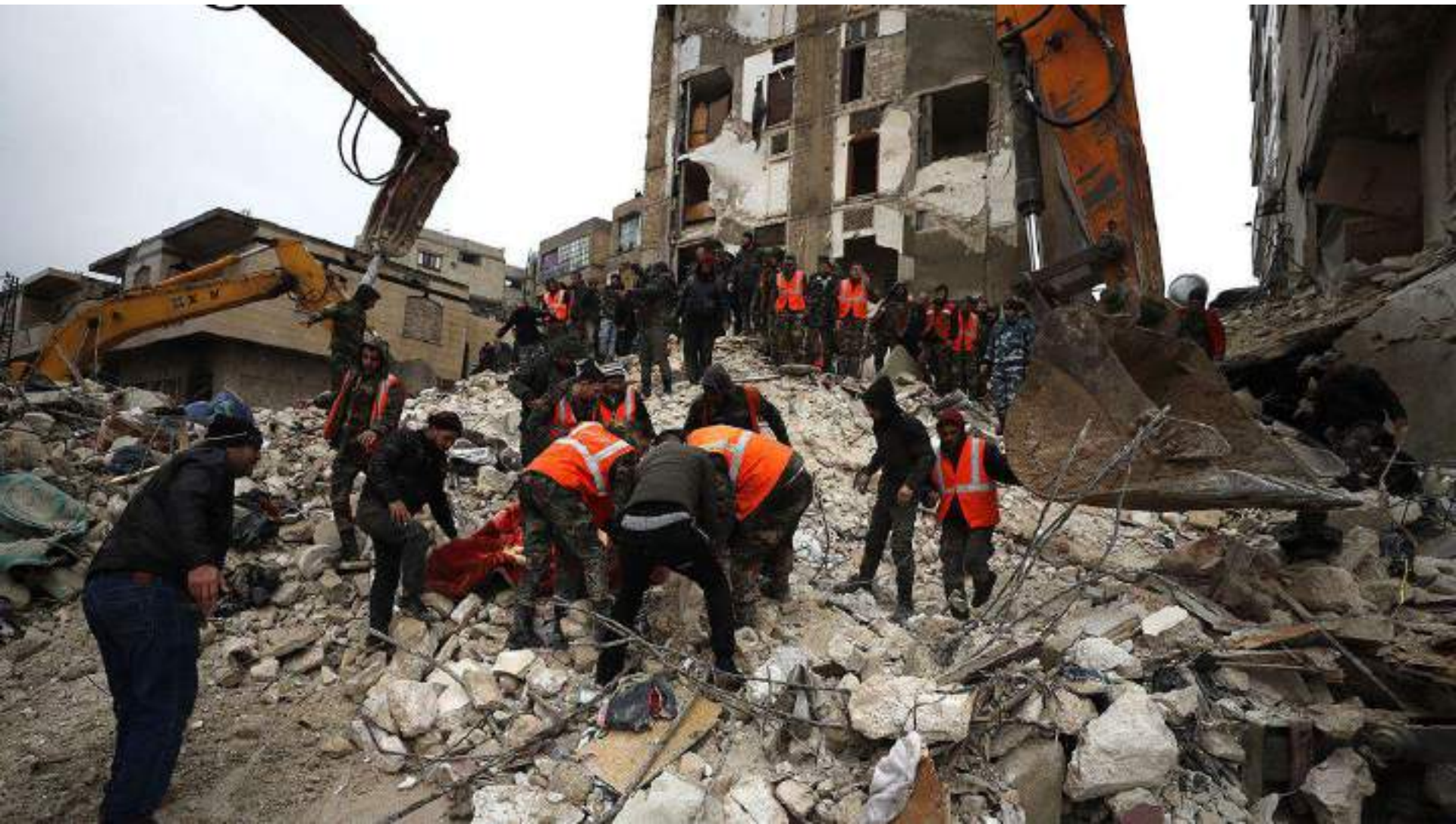
Civil defense workers search through the wreckage of collapsed buildings in Hama, Syria, Monday, Feb. 6, 2023.
